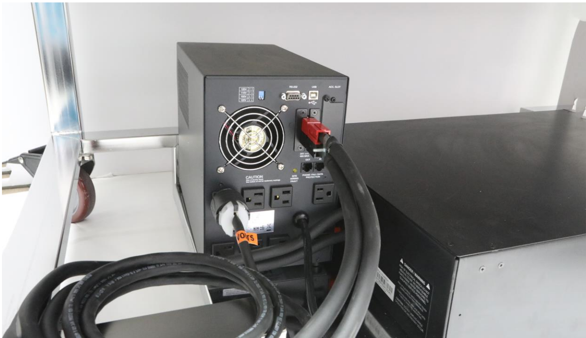
Figure 14. Correct positioning of the UPS and large 3 hour battery pack
