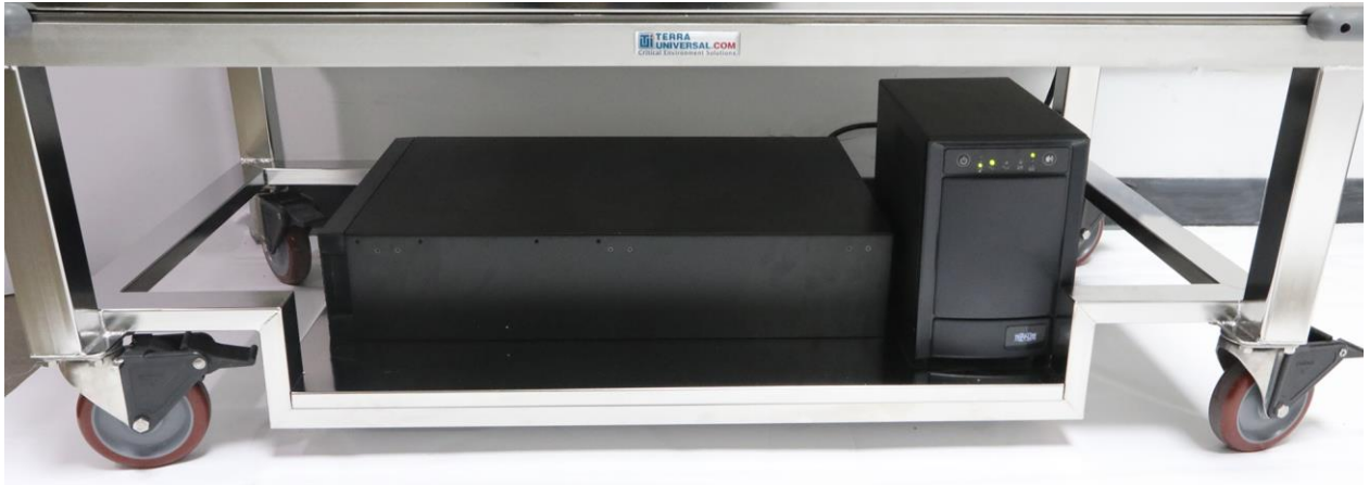
Figure 13. Correct positioning of the UPS and large 3 hour battery pack
