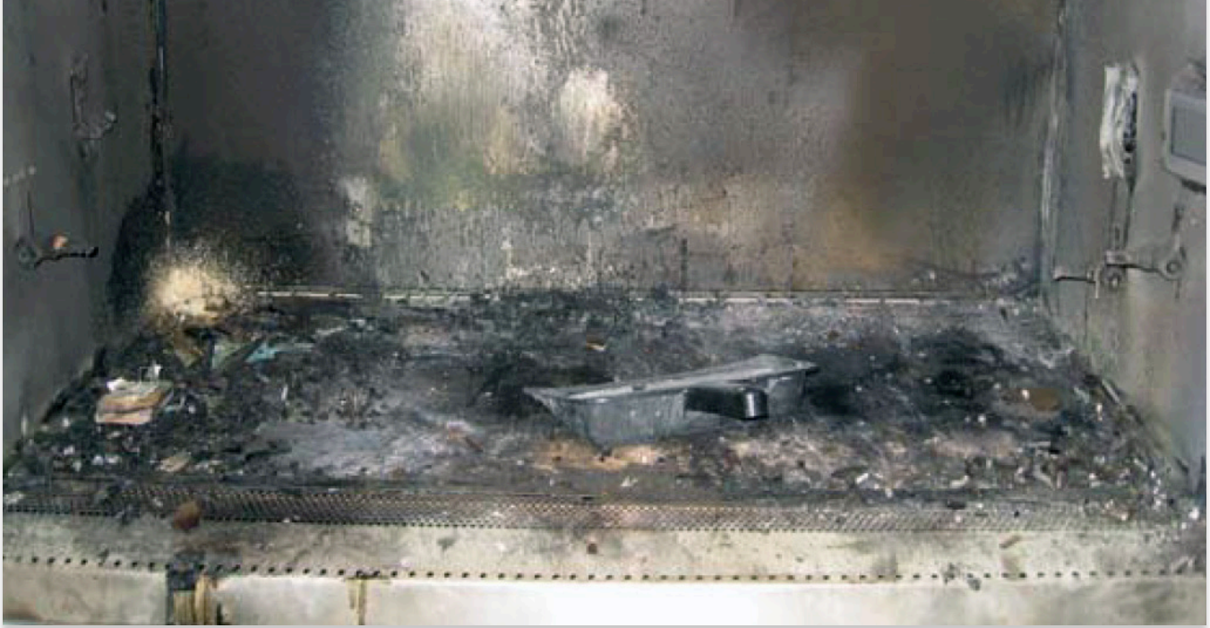
BSC with fire damage
