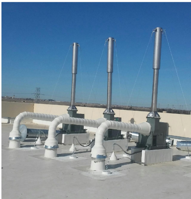
Typical Class II BSC Exhaust System
