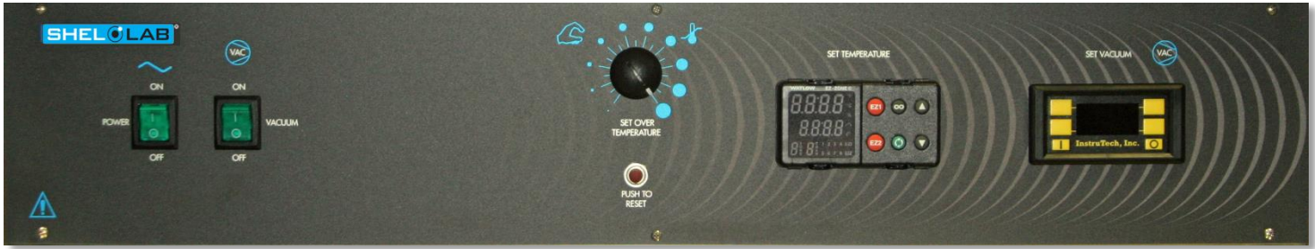
Figure 10: Control Panel SVAC9-2 and Watlow Temperature Controller
