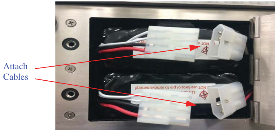
Figure 3-6 Dual-Battery Compartment With Batteries
